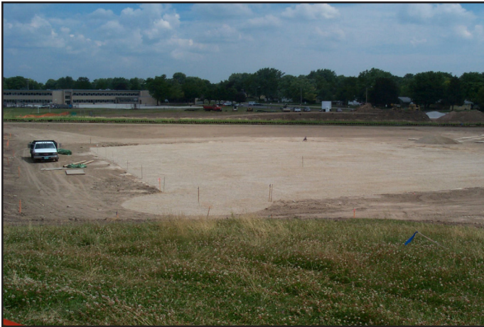
Bare soil during sports field construction - Picture courtesy of Aaron Volkening, P.E.
